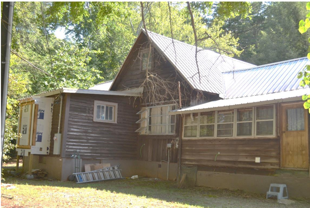
Mitchum-Hensley House, Side (West) Elevation, Bedroom Bay (Left), and Side Kitchen Extension (Right), Looking Northeast.
